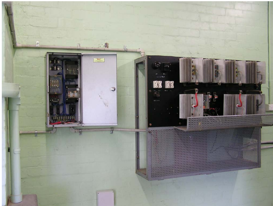
Photograph of a typical TDU installation (old type).
