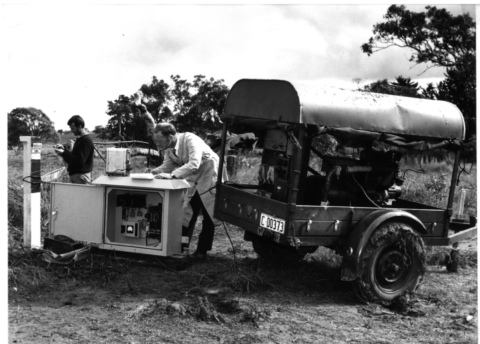
12.12 Carrying Out Temporary CP Testing
