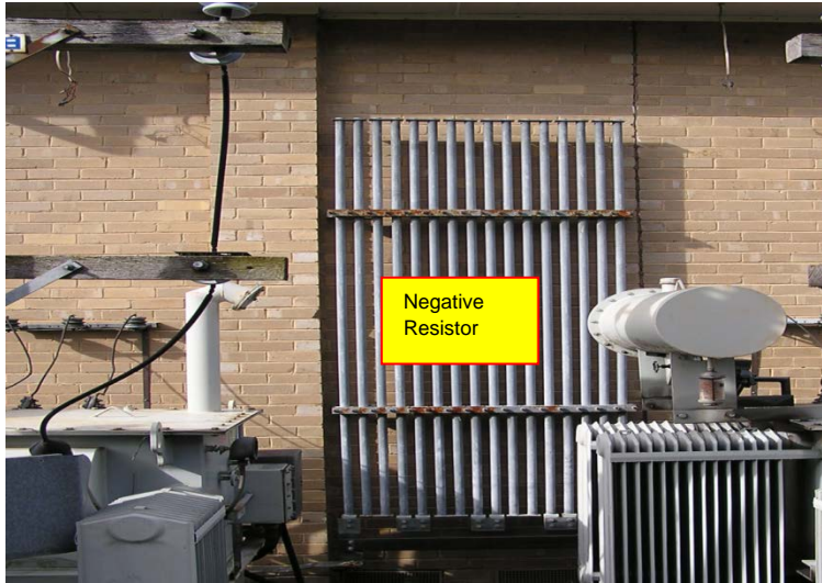
Figure 12 - Typical tramway substation showing negative resistor.
