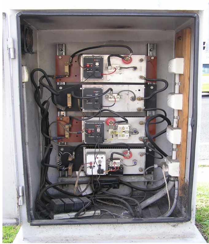
Photograph of typical VCDB installations with DC supply at the substation.
