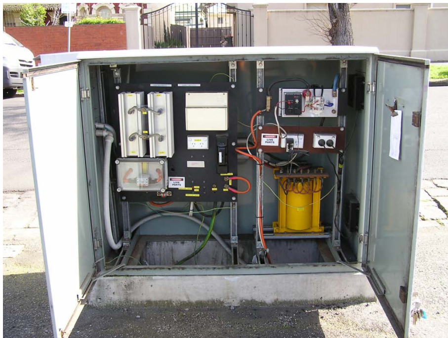
Photograph of typical VCDB installation which includes DC supply.
