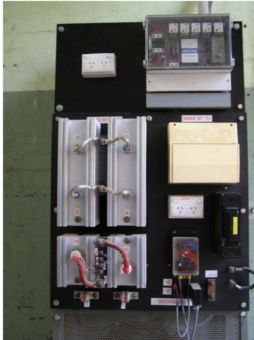
Photograph of a typical TDU installation (new type).
