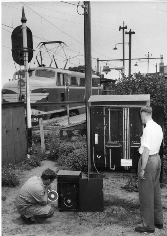
12.13 VR Drainage Bond, Spotswood
