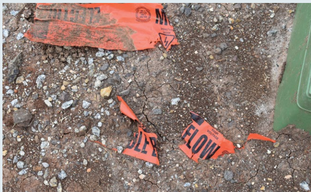
Figure 21: Orange marker tape to provide warning of underground electrical services.
