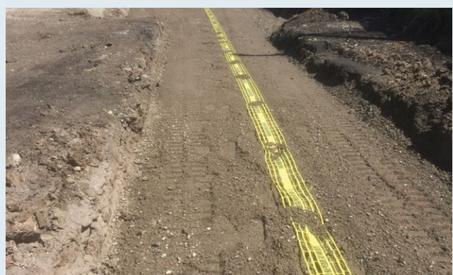
Figure 24: Yellow marker tape in a trench to provide warning of underground gas services
