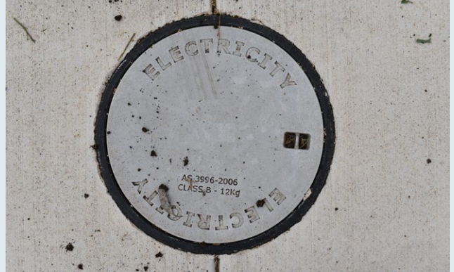
Figure 6: A pit indicating electrical cables below ground.
