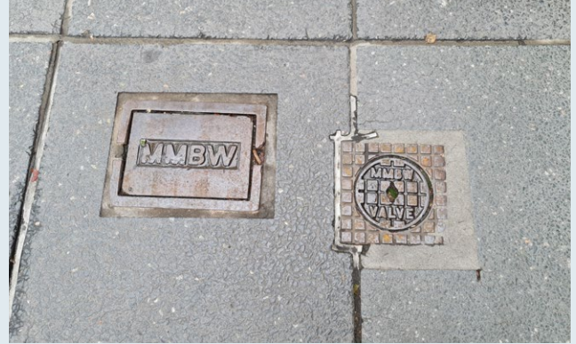
Figure 16: Hydrant connection points and water stop valves indicating water services underneath in close proximity.
