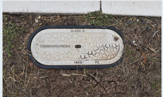
Figure 18: A pit indicating that there are telecommunication cables below ground.
