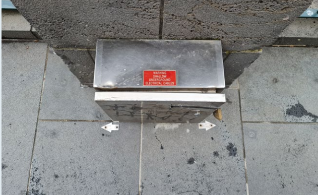
Figure 5: An electrical connection box providing warning that there are shallow underground electrical cables. Two arrow indicators showing the direction of the cables.
