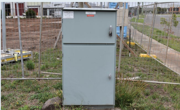
Figure 9: A customer switchboard and supply point for an electrical installation on private property.
