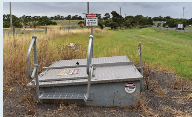
Figure 14: A warning sign and an access pit for underground high pressure oil pipeline.
