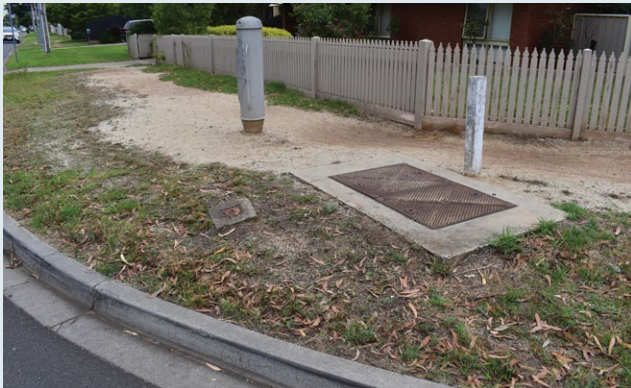
Figure 17: A telecommunication riser and pit indicating the presence of telecommunication cables in vicinity.
